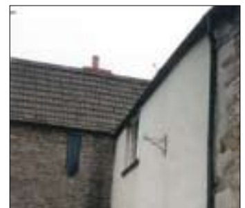
Stone quoins incorrectly expressed separately from the render. The render should be swept over the corners of the building, with no quoins.
